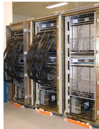
The APEmille installation at DESY Zeuthen. Each rack hosts 256 nodes.
